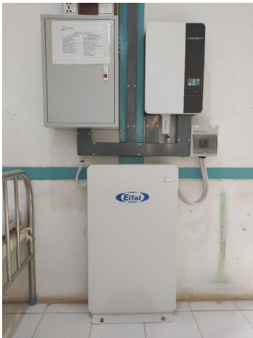
Panel Box, Inverter & Battery
