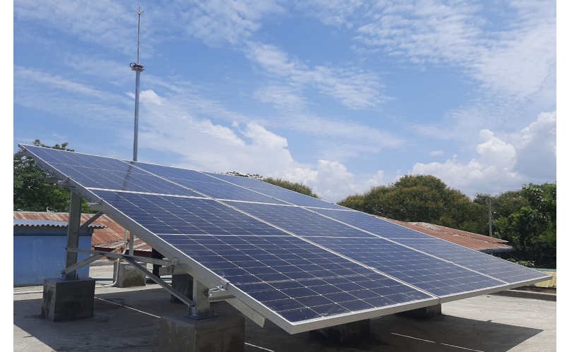
PV Module Capacity (575Wp x 6 Module)
