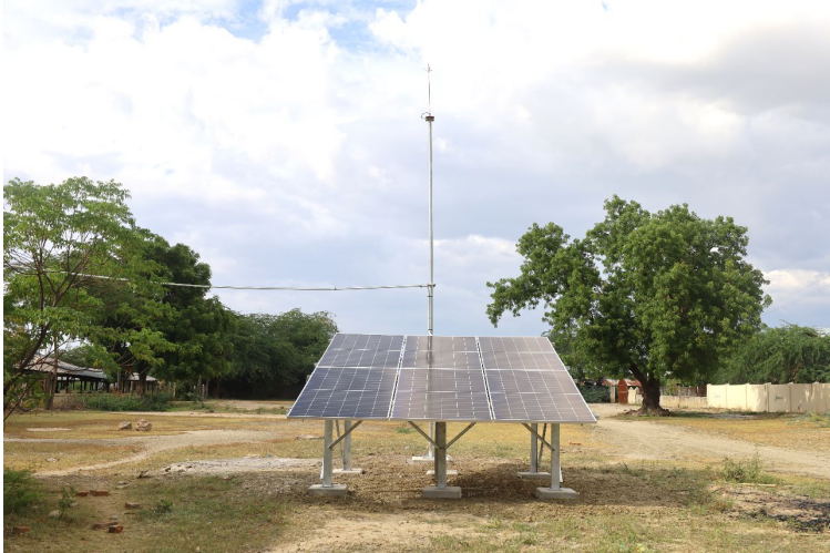
PV Module Capacity (575Wp x 6 Module) Ground Mounted
